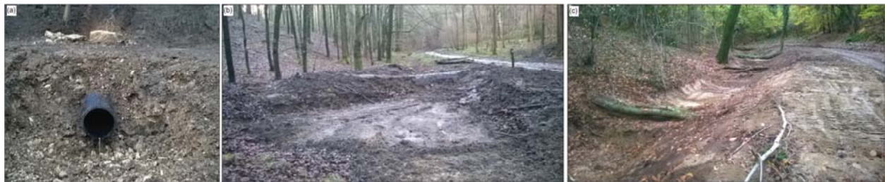
Figure 6: Examples of the culvert and grip interventions that have been implemented in the Stroud Frome Catchment to reduce surface runoff and material transportation from tracks (a) large culvert pipe and stone soak away in a catch pit under the inlet pipe, (b) a track-side storage area (c) grip created alongside tracks
