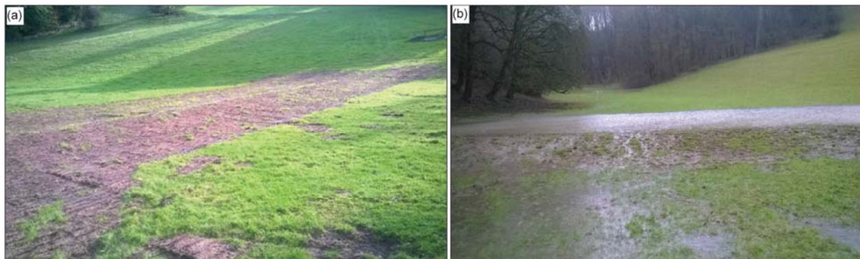
Figure 5: An example of an earth bund installed in the Stroud Frome Catchment, (a) immediately post-construction and (b) retaining water during storm event
