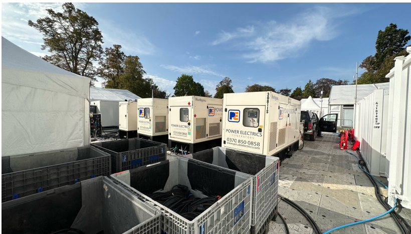
HVO Generators used to power refrigeration
