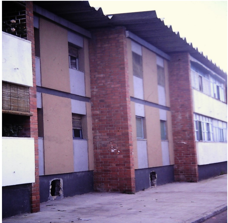
Figure 19. Housing in the San Cosme UVA in 1978, showing the holes knocked through the egg-box structure to facilitate ventilation and drainage of the cellar. Photo: M. Wynn.
