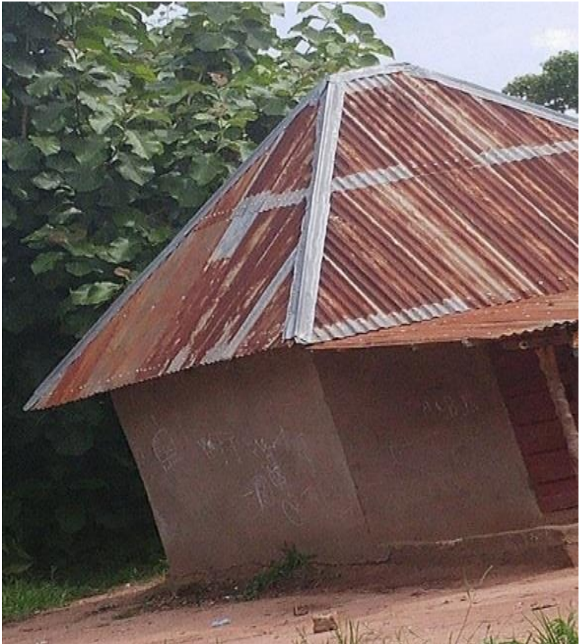
Figure 6.18: Plastered mud/concrete walls with zinc roofing sheets Farmers do live with grains in this type(live-in). Credit: Author from the field.
