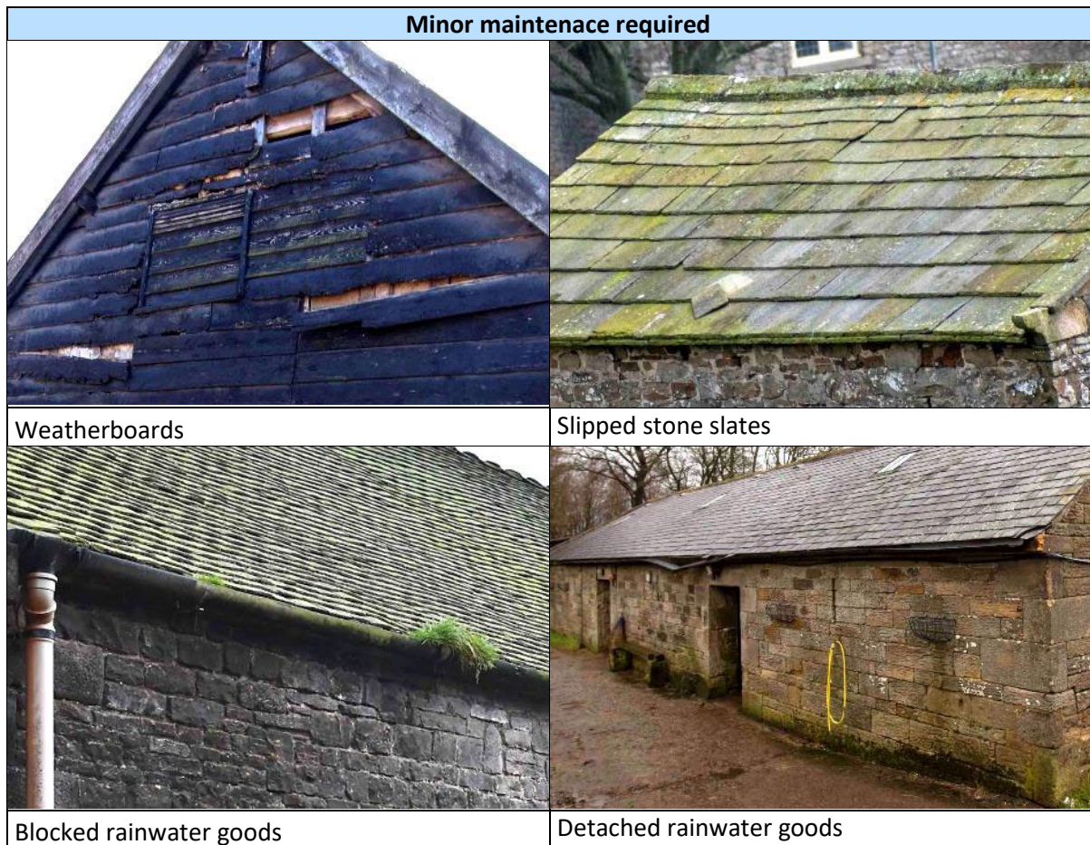
Figure 3.5-40 Minor maintenance required
