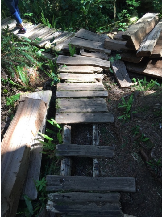
Figure 6 – Big Tree Trail damaged boardwalk section
