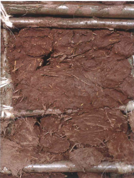
Fig.44 Shelter: external surface showing holes through to interior
