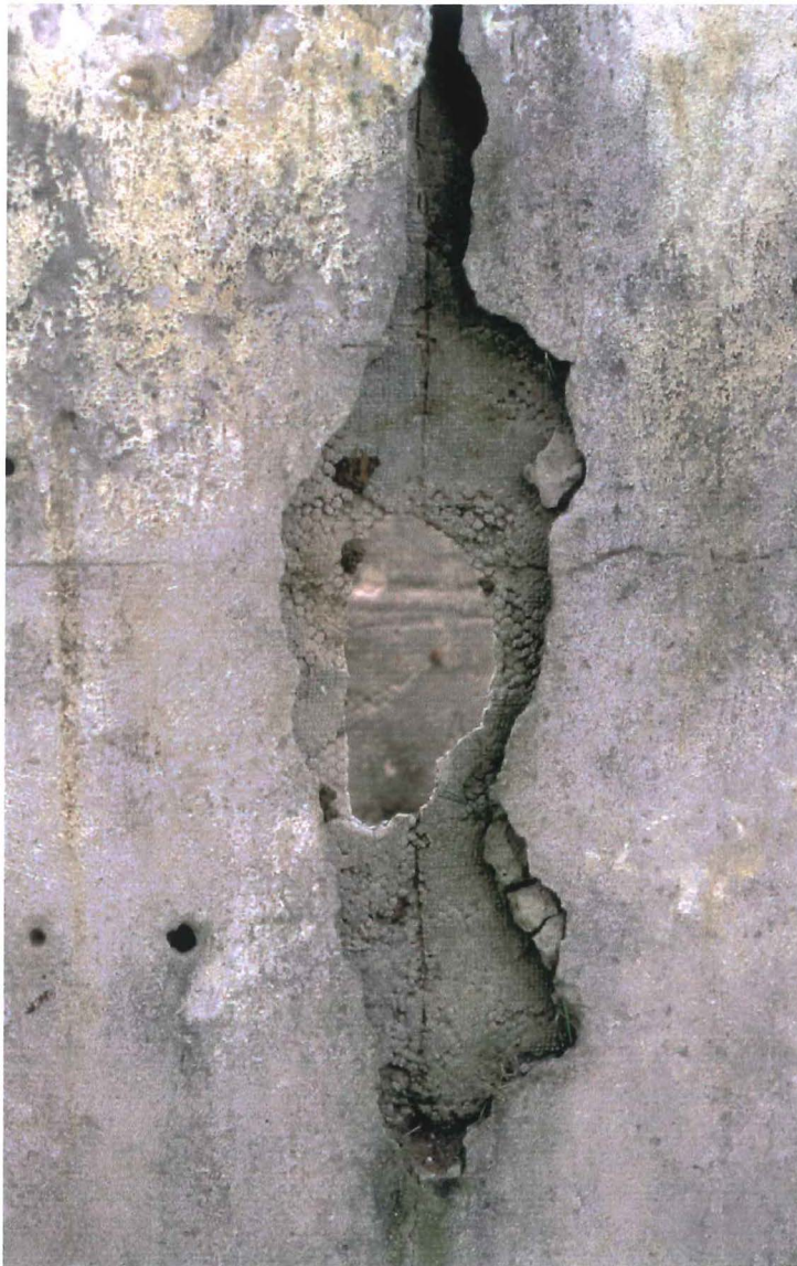
Fig.22 Detail of Mission house wall showing casting technique using sewn flour sacks, chickenwire reinforcement and cement, creating a cavity wall
