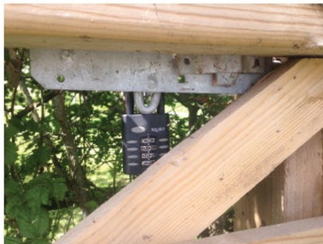
Figure 7 New gate for closing the road during floods. Image: Ricketts, 2018.
